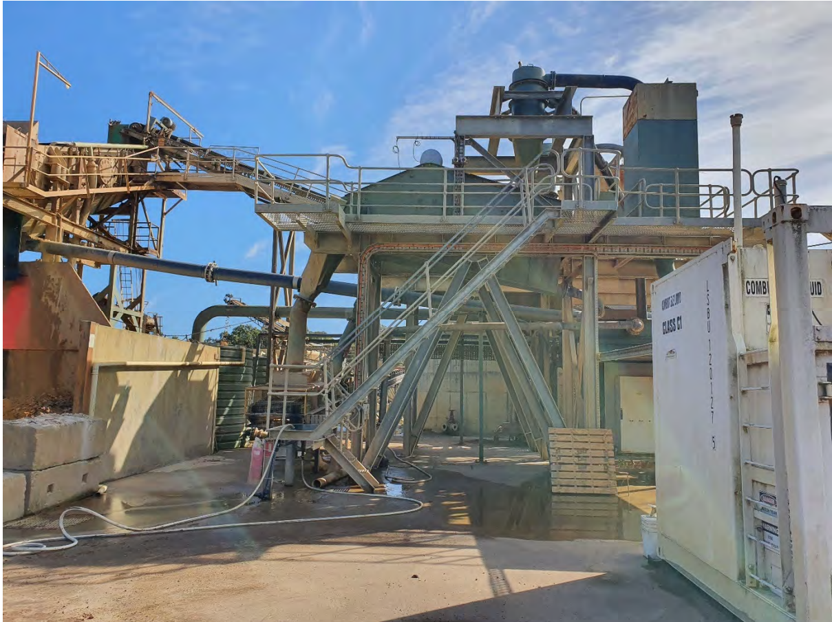
Processing Facility with Screen
