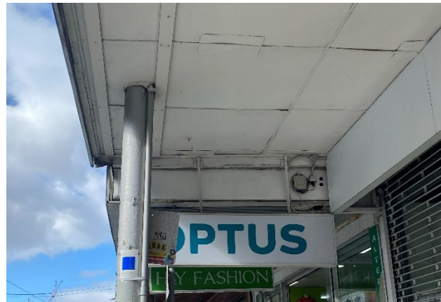
Figure 3-25. Overhead pole through the awning at 143-145 Hopkins Street, facing east
