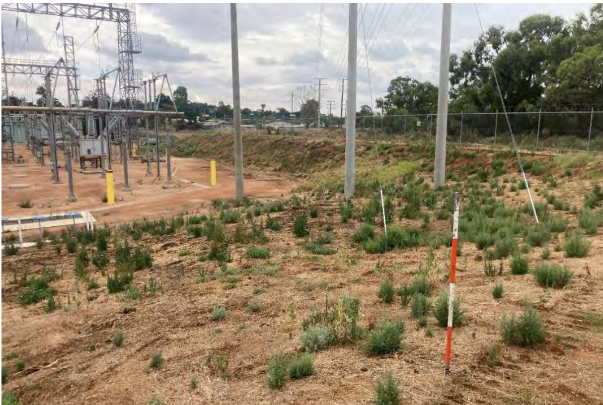
Figure 4 Levee surrounding the site which is ~3m below natural ground (Source: Red-Gum Environmental Consulting Aboriginal Cultural Heritage Due Diligence Assessment)
