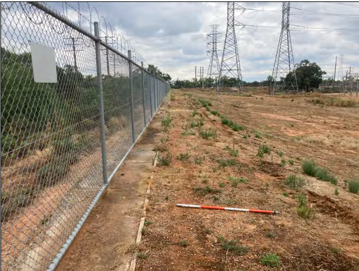
Photo 6: Two new 220kV poles to be developed along fenceline, north east boundary of site. Photo: D.Wall, 2023.
