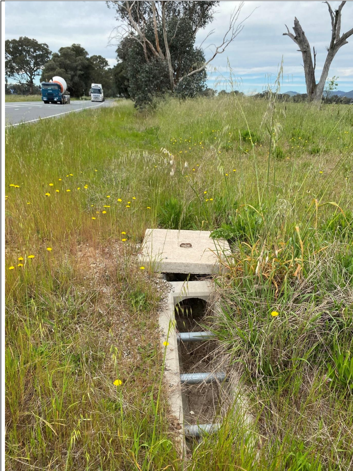
Culvert along Murray Valley Highway facing east (corner of Barnawartha -Howlong road)
