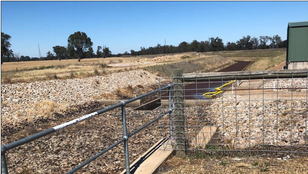
Figure 9 Winton Wetlands Infrastructure (holds rainwater runoff)
