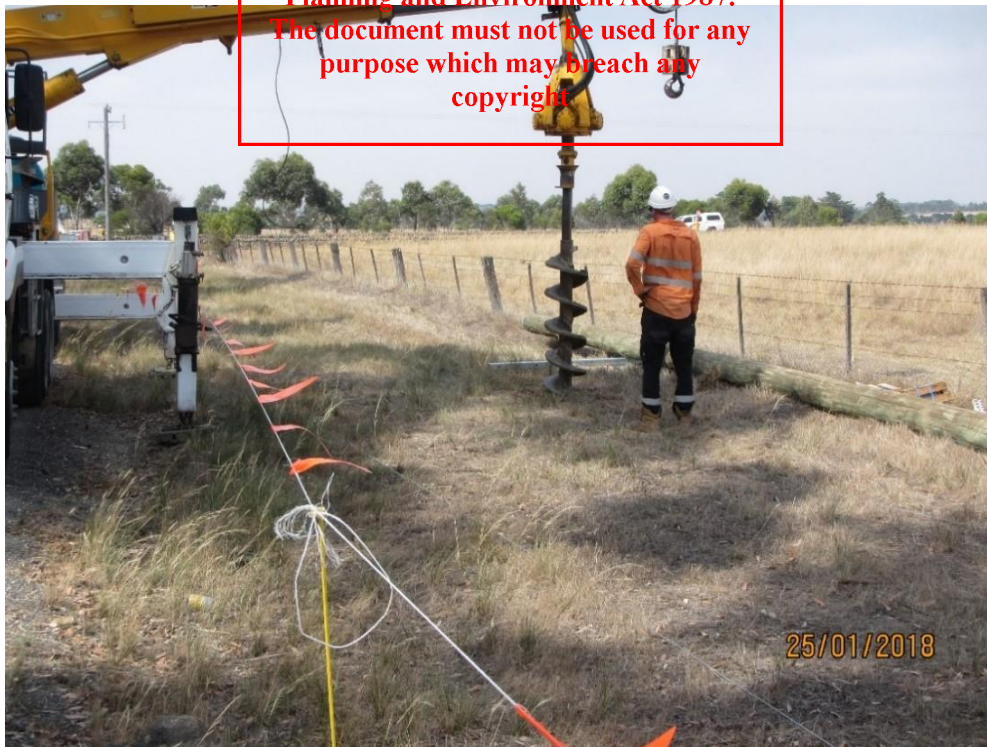
Figure 3. Example of a truck arm remaining on road verge to auger a hole
