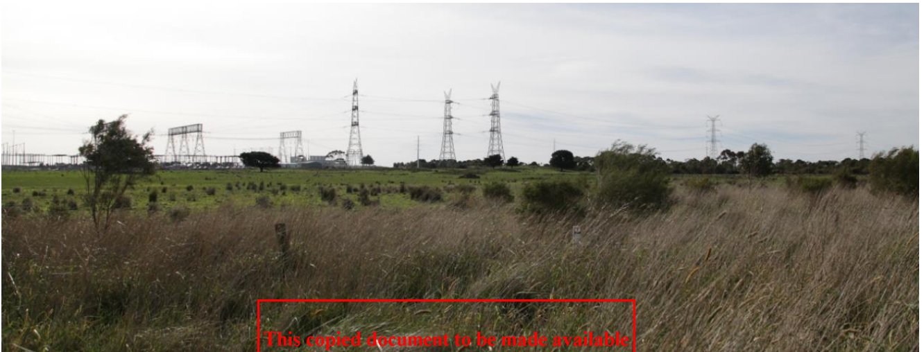
Figure 6-2 Existing Tarrone Terminal Station and 500kV transmission lines
