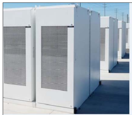
Typical Battery storage unit
