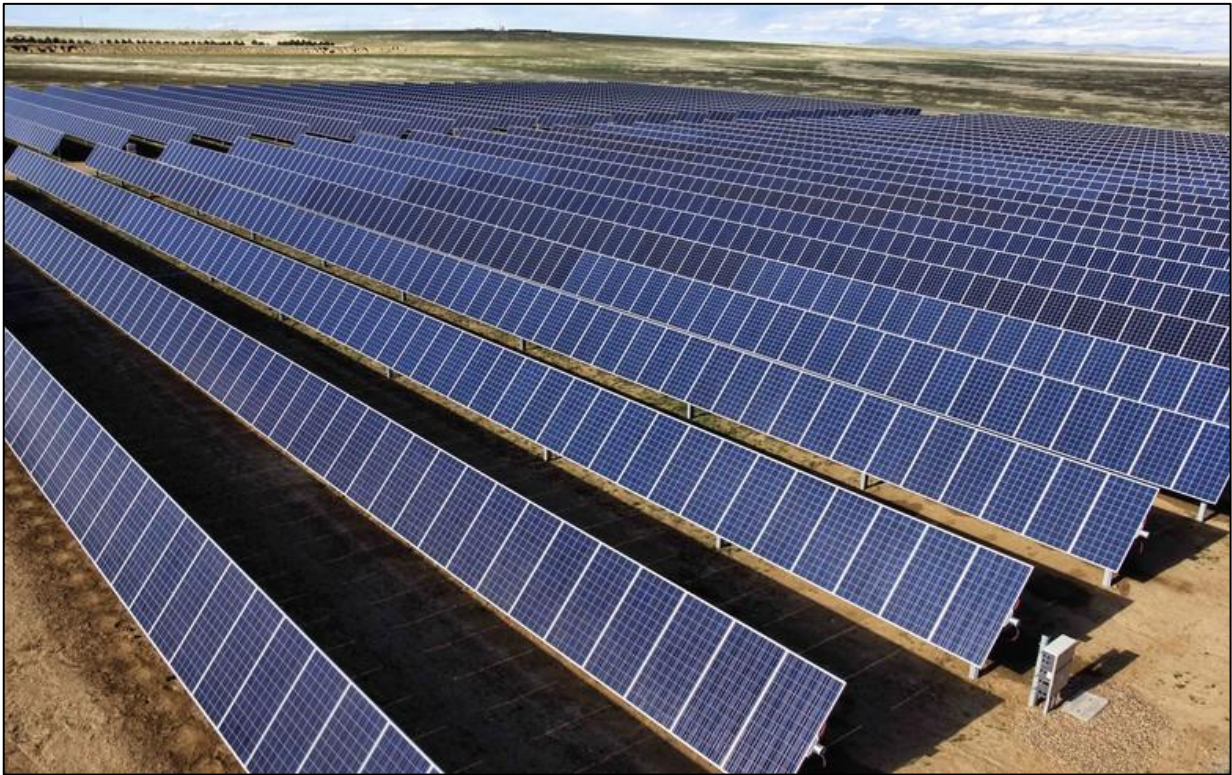
Figure 7. Example of a single axis tracker PV system at 60° angle with maximum inter-row shading.
