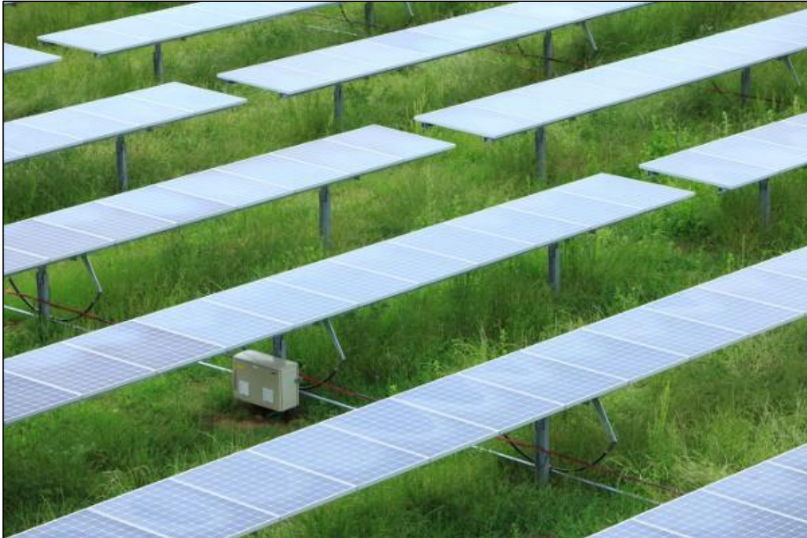
Figure 4. Illustrated example of vegetation growth below a single axis tracker PV system.
