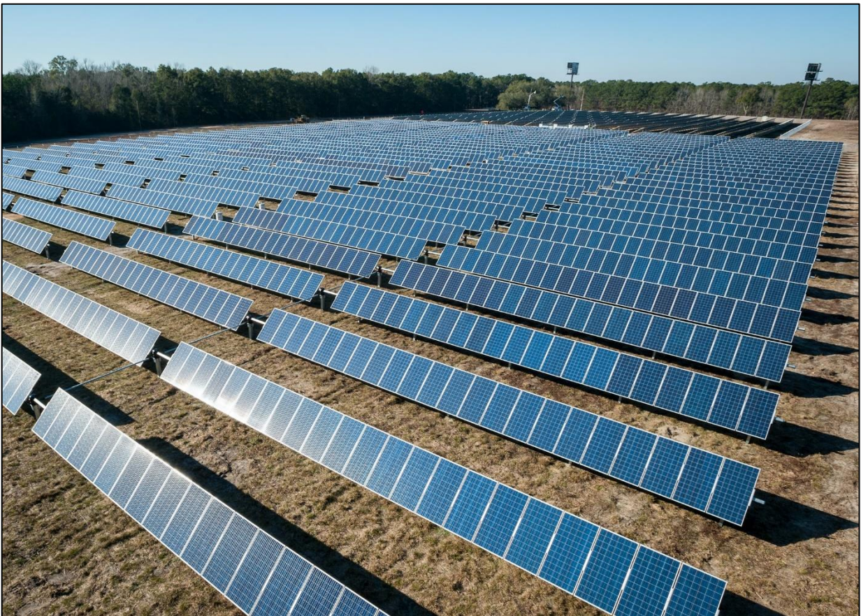
Figure 8. Example of a single axis tracker PV system at 40° angle with reduced inter-row shading.
