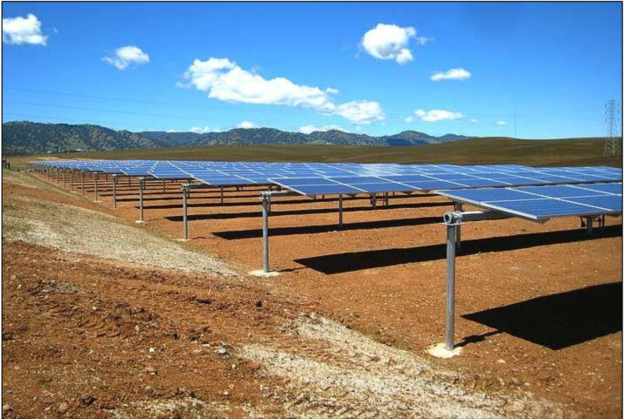
Figure 9. Example of a single axis tracker PV system at 0° with zero inter-row shading.
