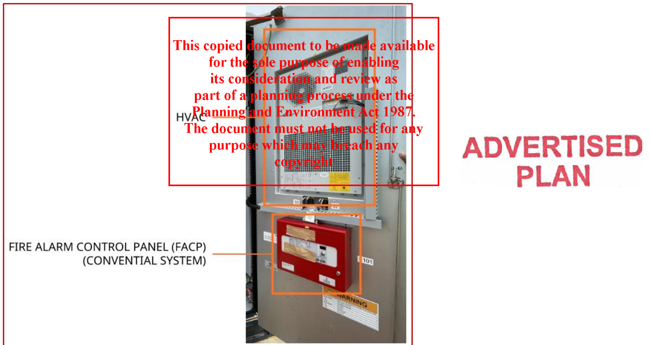
Figure 7: Fire alarm panel on the GridSolv Quantum DC door
