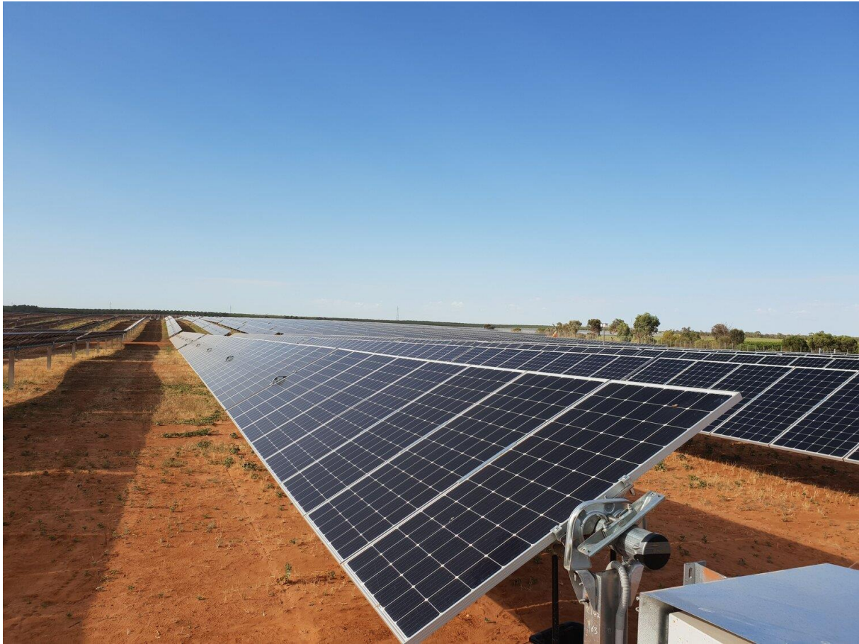
Figure 11 Example of Typical Single Axis Tracking System (Source: Wemen Solar Farm)
