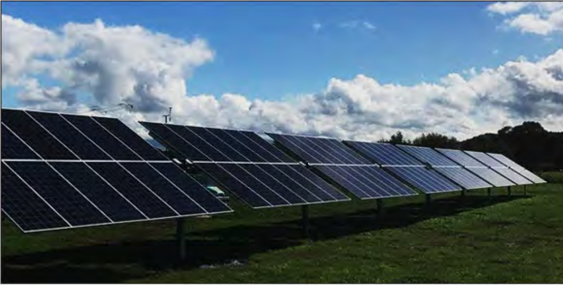
Figure 3-2 Example of a single axis tracking system
