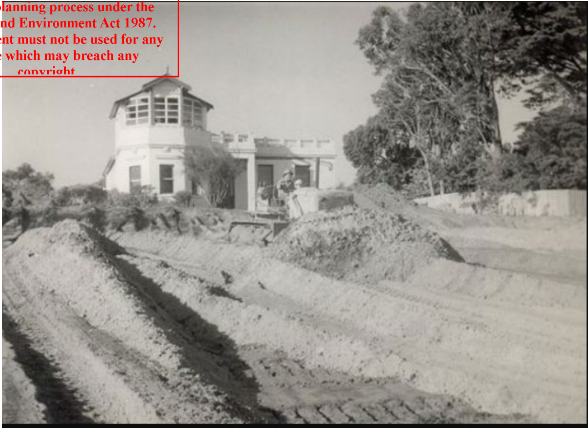
“Bay View” with a bulldozer in the foreground excavating the Junior School oval – probably late 50’s
