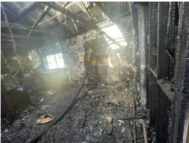
Figure 8: Fire damaged internal timber walls.
