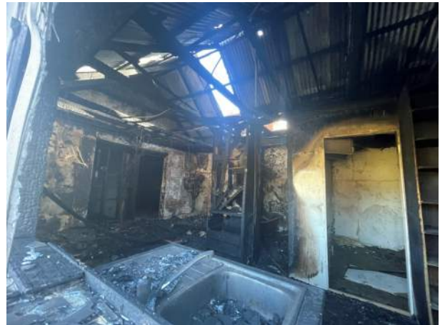
Figure 3: Condition of fire damaged part of existing building.
