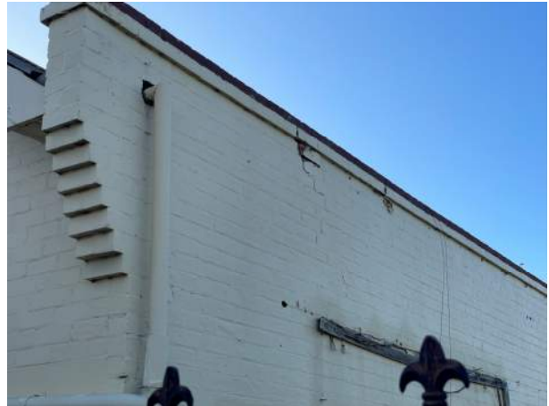
Figure 13: Cracks in masonry wall.
