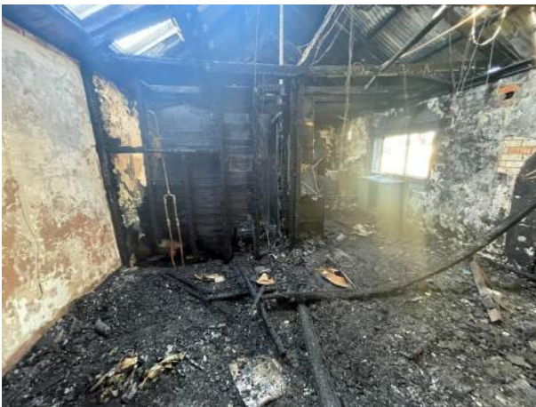
Figure 4: Condition of fire damaged part of existing building.
