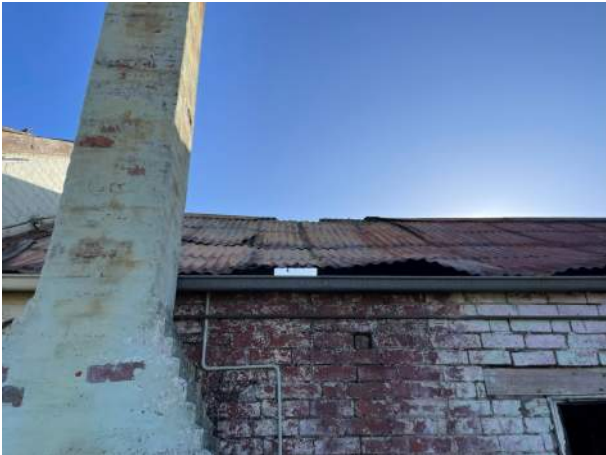
Figure 12: Cracking and mortar loss in masonry walls.
