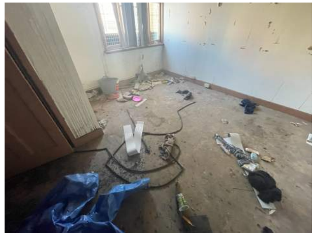
Figure 5: Vandalised part of existing building.
