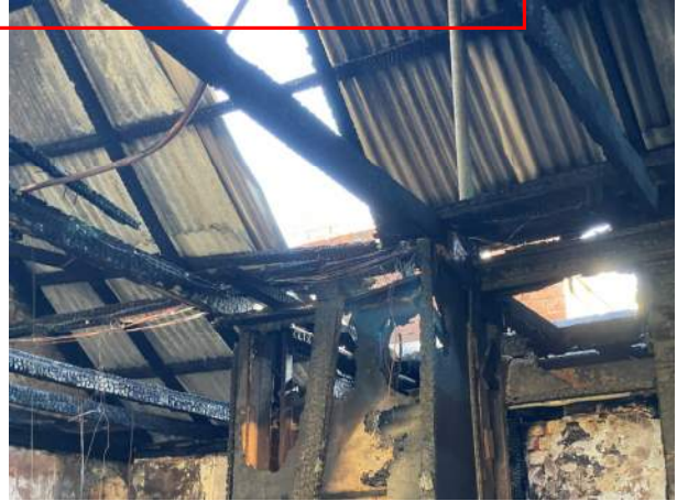
Figure 7: Fire damaged timber ceiling joists.
