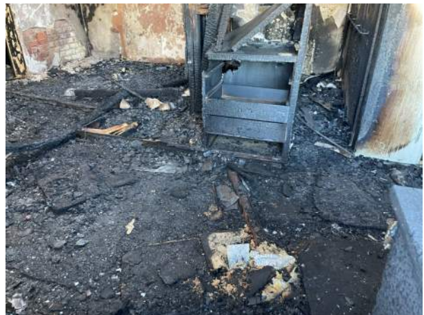
Figure 9: Fire damaged timber subfloor.
