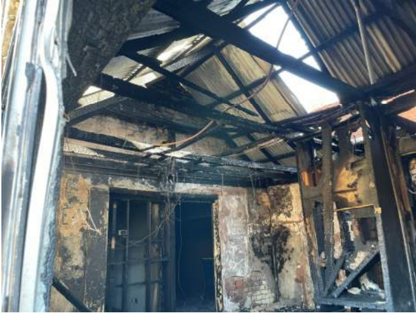
Figure 6: Fire damaged timber roof rafters.
