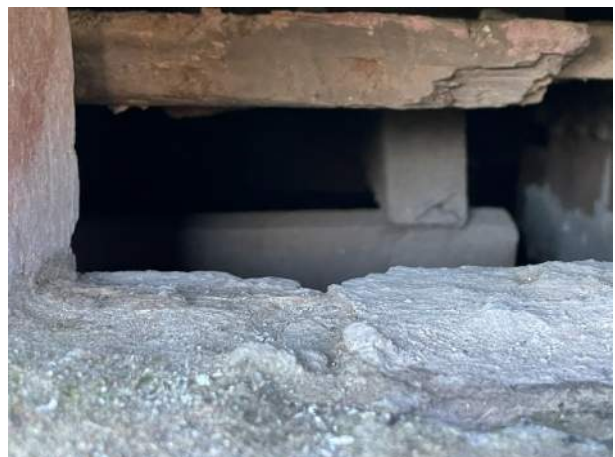
Figure 11: Timber subfloor condition.
