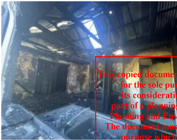
Figure 12: Fire damage to rear part of the building. Source: SCE Australia, 2025
