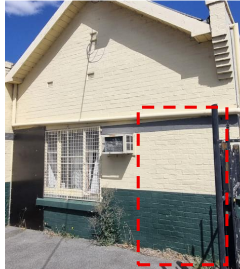
Figure 19: Different brick texture suggests patch infill of former opening. Source: Trethowan, 2025.
