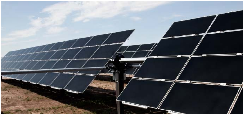
Plate 1. Example of a typical frameless solar array mounted on a single axis tracking system 10
