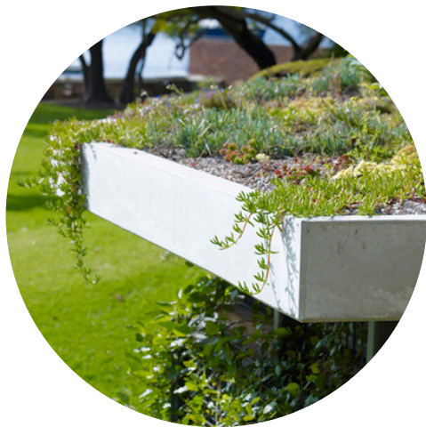
Semi-extensive roof planting
