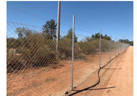
TYPICAL GALVANIZED FINISHED MESH FENCE
