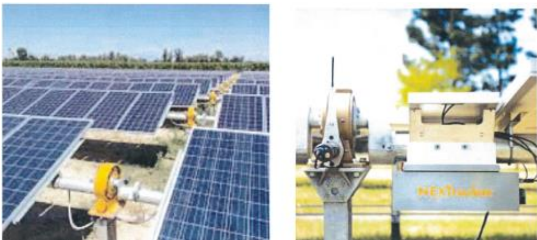
Figure 1. Typical solar tracking system and motor (equipment manufacturer subject to change)
