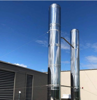
SSF - STAINLESS STEEL FLUES PAINTED
