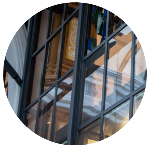
Contemporary Monument aluminium framed windows creates continuity between the podium and tower.
