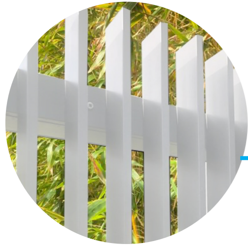
Vertical white metal balustrading to upper level balconies of podium, enforcing a different architectural style between podium and tower.
