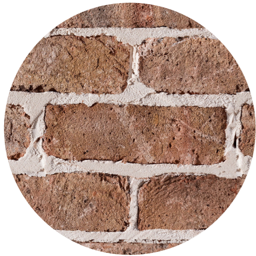
Brick Tiles Robertsons Rustic Red brick tiles at ground and first floor Front facade podium levels. Brick attached to precast concrete panels walls.
