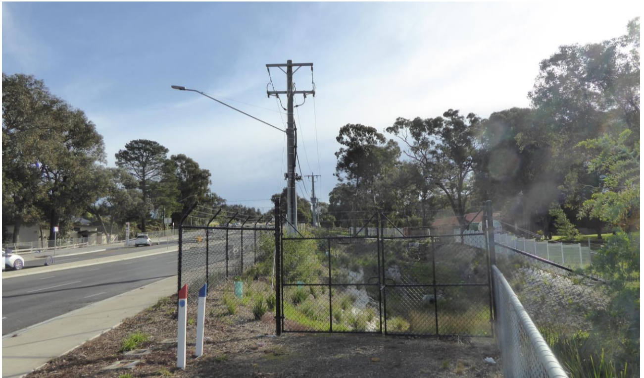
Figure 17 Existing electricity distribution infrastructure in Yan Yean Road reserve, to the west of the site entrance
