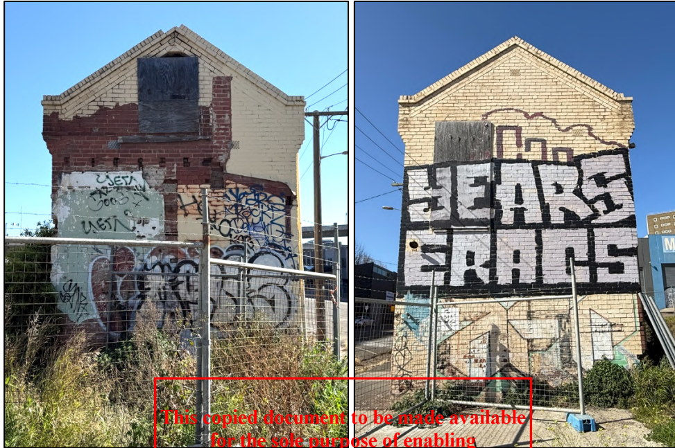
Figure 13 (left) View of the east elevation showing boarded up first floor opening (right) The west elevation showing original triangular first floor window opening (now boarded up)
