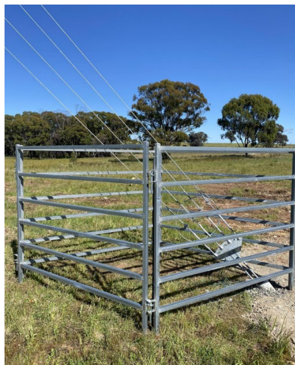
Photo 3.11 Example of a guy wire attachment
