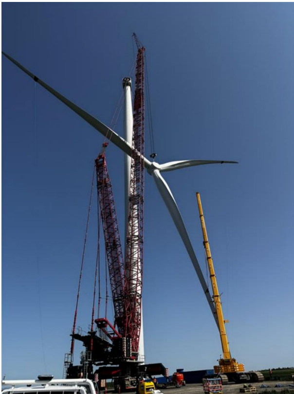
Photo 3.5 Example of a WTG Tower with the Nacelle and Hub at Murra Warra Wind Farm (Vic)
