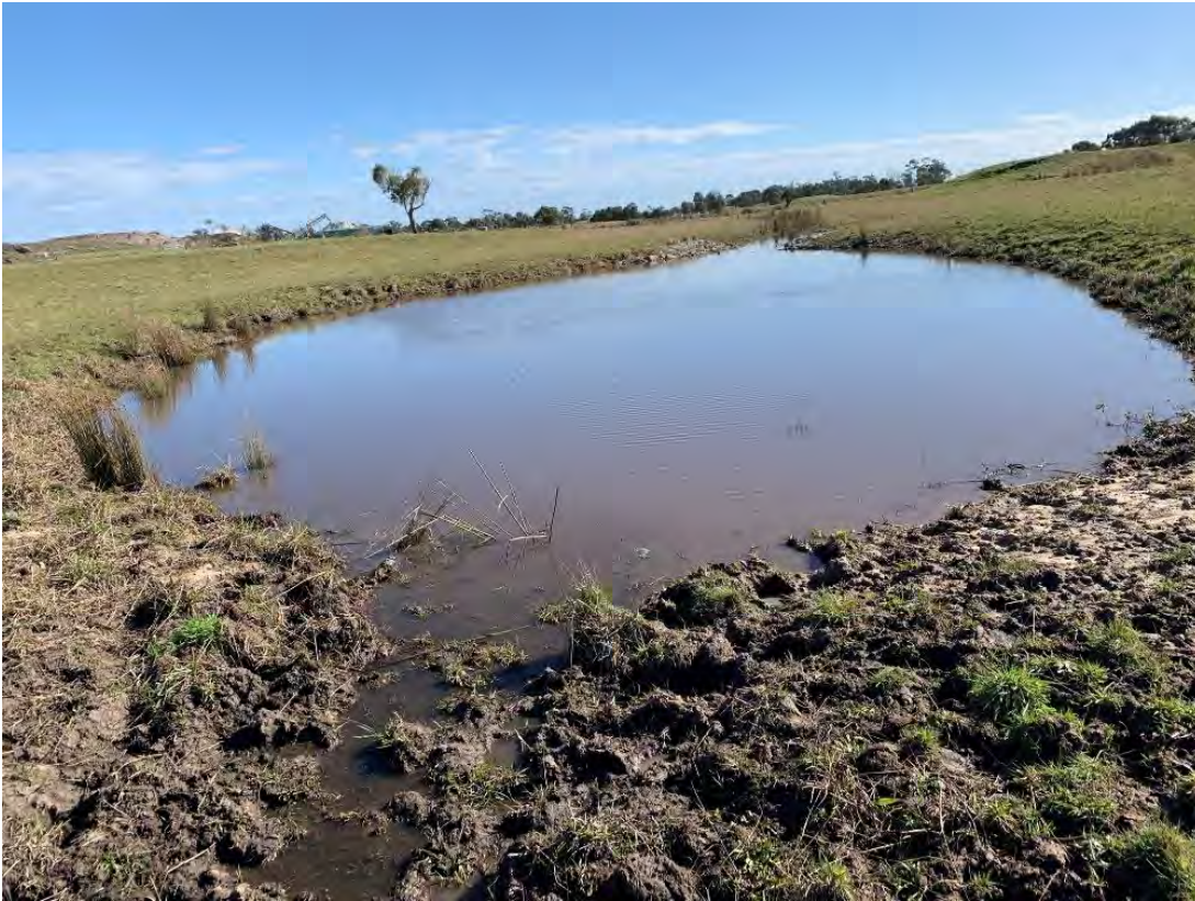
Figure 3.4: Typical chain of ponds at Reach A showing signs of bank instability
