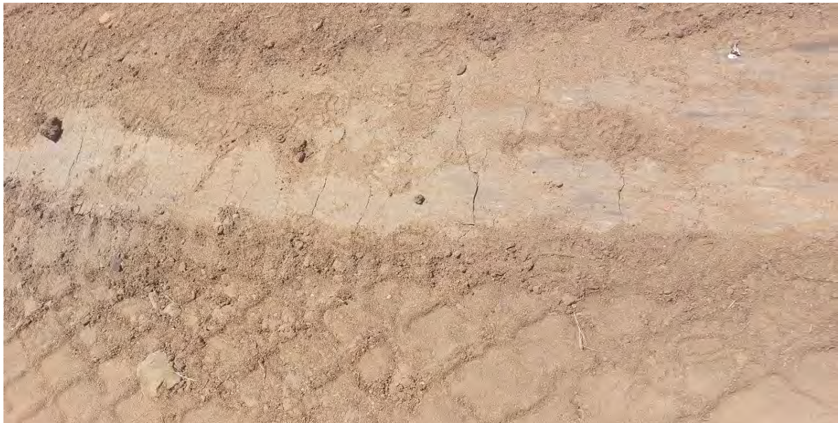
CPT-03A - SURFACE CRACKING - 12/01/2023
