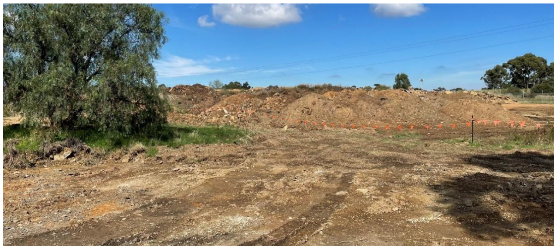
Figure 30 – Soil heaps resulting from major earthworks observed during site walkover (Source: DJAARA, 2026)
