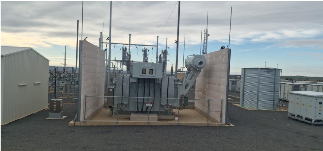
Figure 25 - Noise wall around Clements Gap BESS Transformer (source: Pacific Blue)
