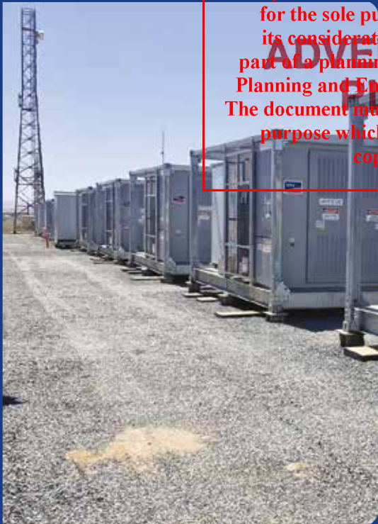
Clements Gap BESS, Pacific Blue's most recently completed battery project
