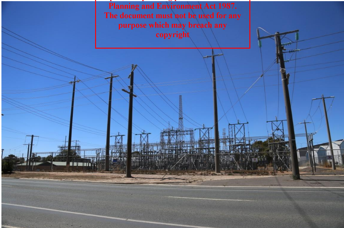
Figure 14 – The Bendigo Terminal Station, as viewed from Allingham Street.
