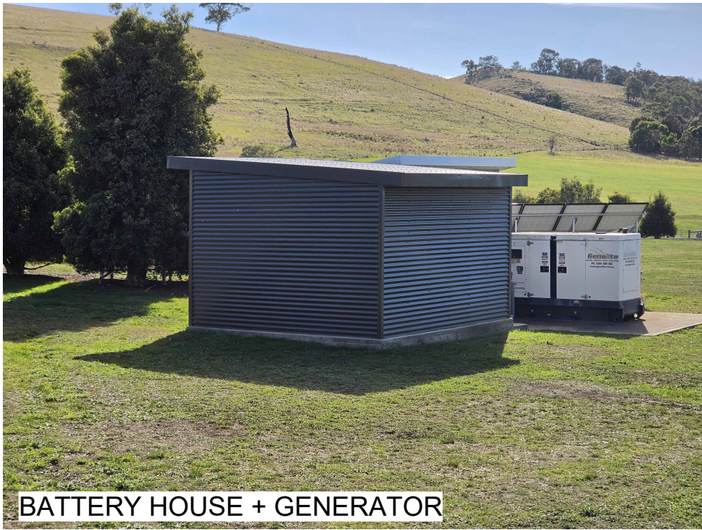
BATTERY HOUSE + GENERATOR
