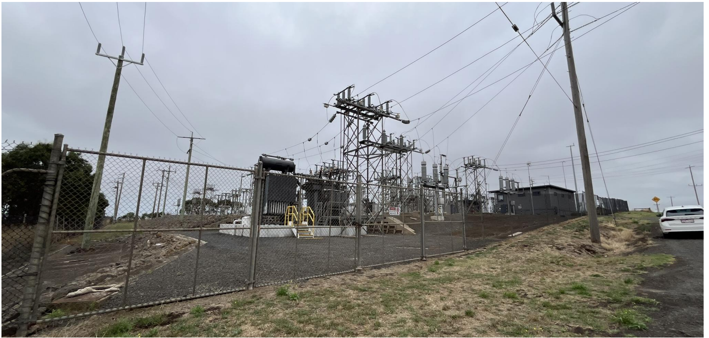
Figure 4: View of the adjacent Koroit Zone Substation. Photo taken from Tower Hill Road on 2 March 2026.
