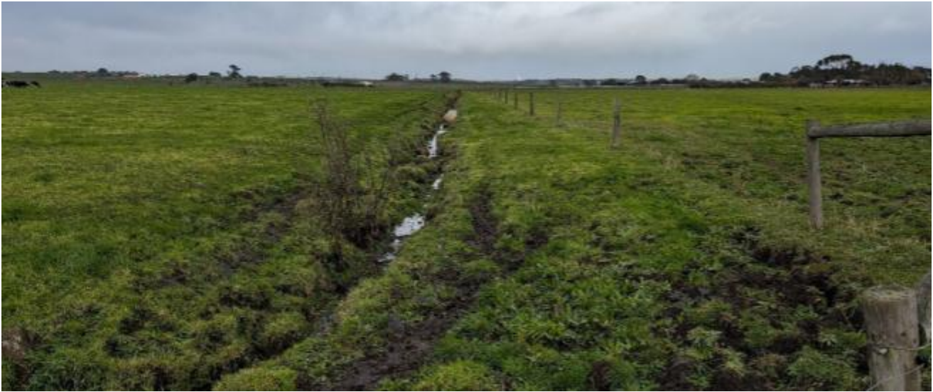
Figure 11: Photo of the drainage line condition, Aurecon 2024.
