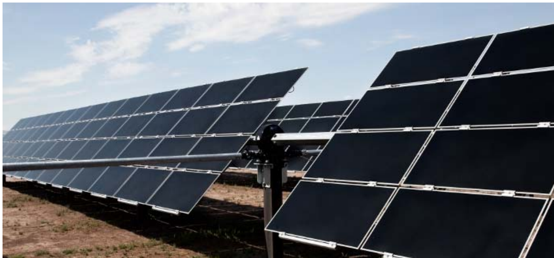
Plate 1. Example of a typical frameless solar array mounted on a single axis tracking system 9
