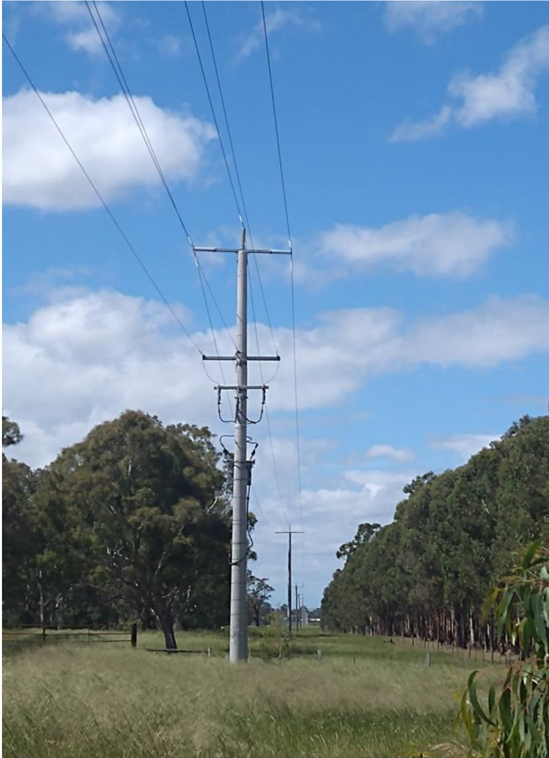
Fig: Point of grid connection at Maffra site
