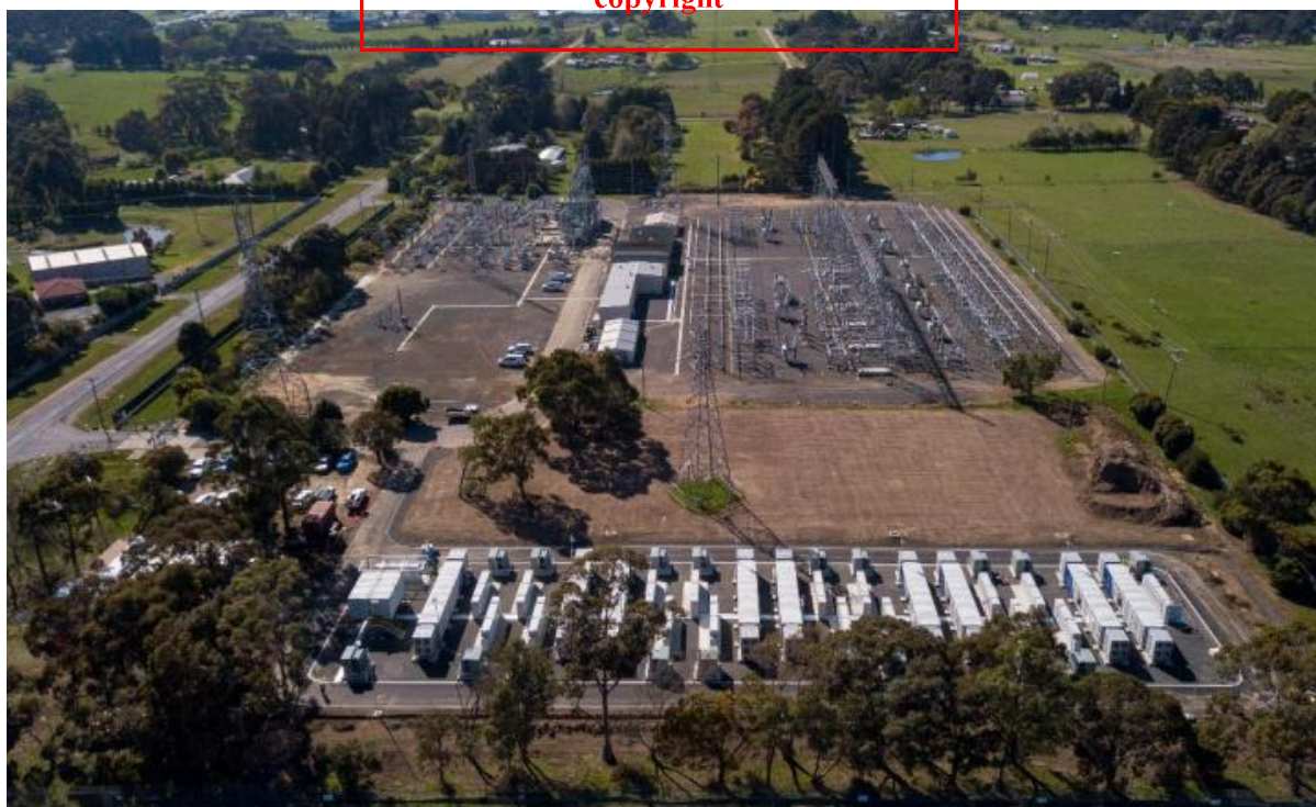
Figure 13 Example BESS Installation
