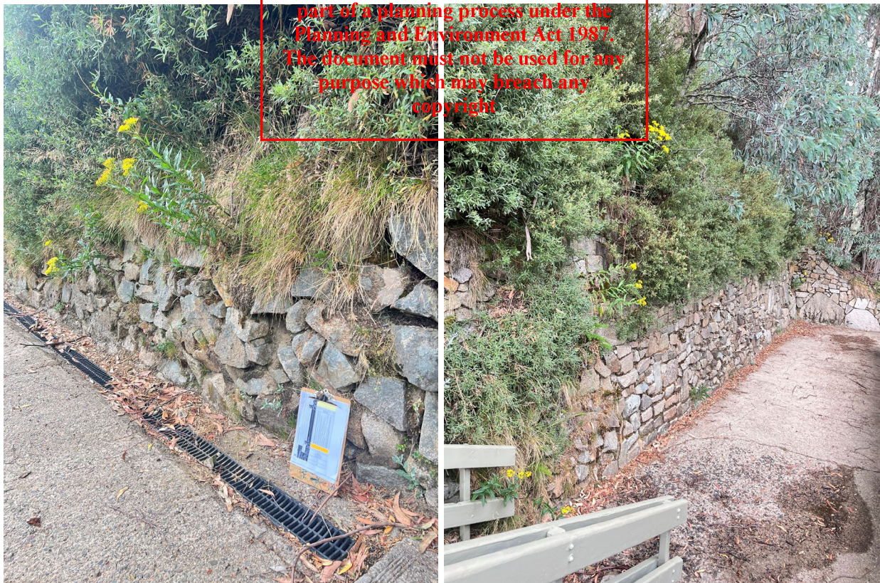
Figure 5 Dry wall downslope of proposed zipline landing structure. Minor blocks dislodged, some sections grouted with drainage pipes.
