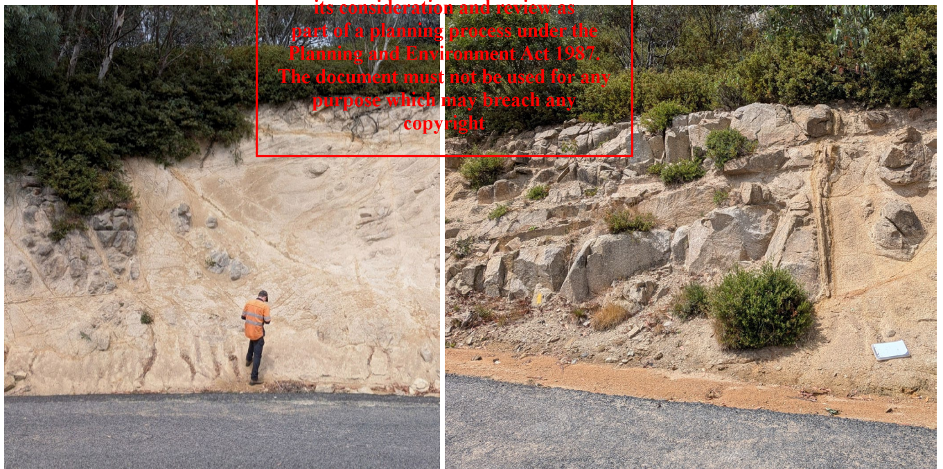
Figure 8 Variable weathering profile of the granodiorite observed at Horse Hill Carpark. Left – extremely weathered soil profile to ~10m. Right – variable profile of Highly weathered to extremely weathered soil profile.
