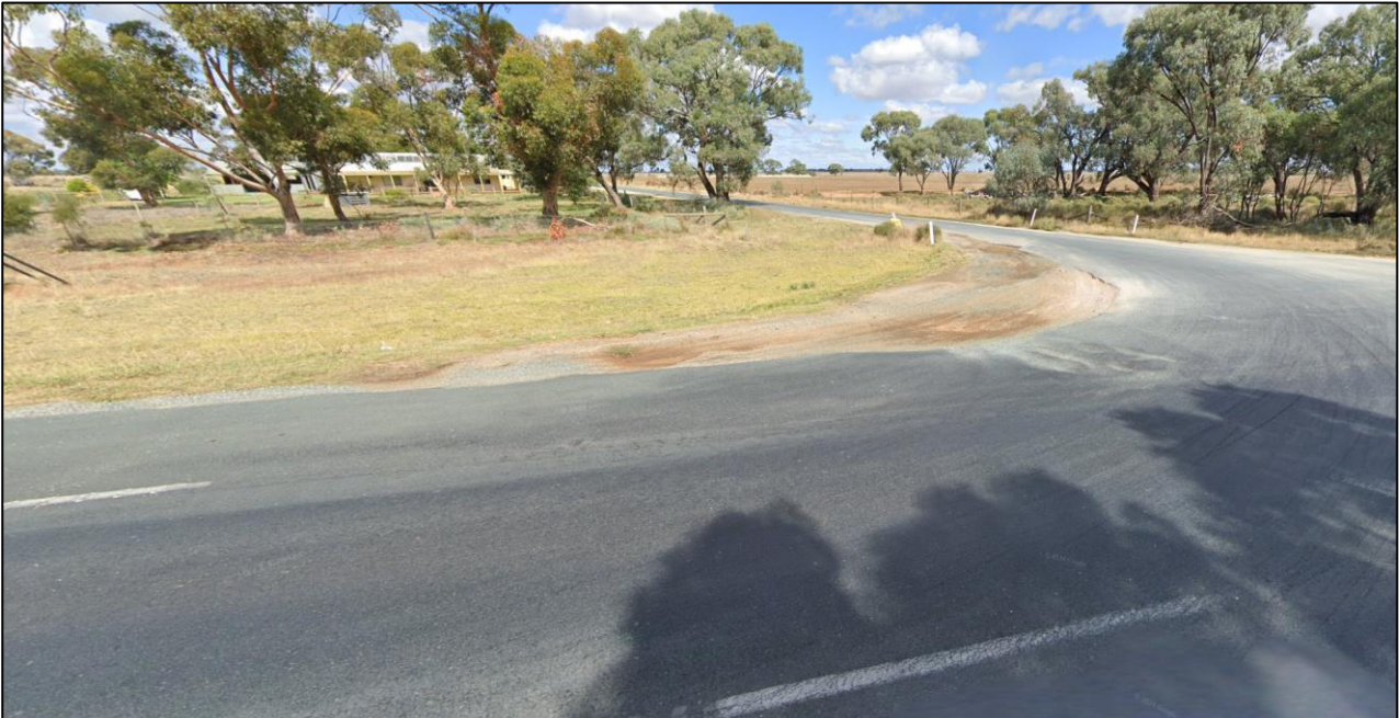
Figure 8-7: Evidence of vehicles tracking over verge at Davis Road turnout
