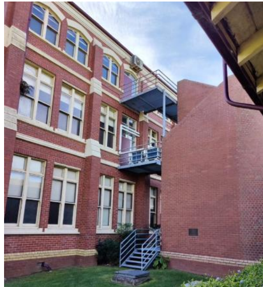
Figure 12: View of the south façade of the South Wing, connected to the external staircase by a work platform. Source: Trethowan Architecture, 2023.
