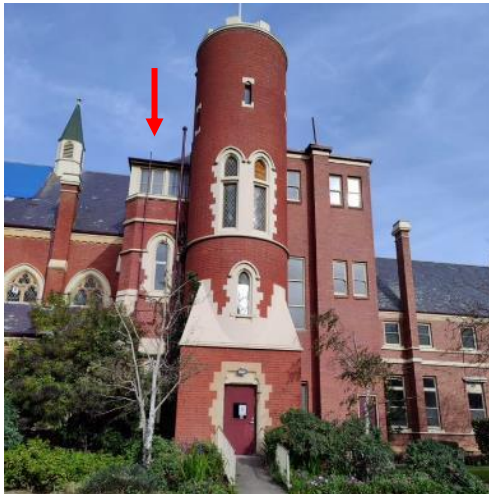
Figure 9: View of the north façade of the Chapel stair tower and adjoining Sunroom to its east (indicated in red). Note the damaged roof, covered in blue tarp, in the far left. Source: Trethowan Architecture, 2023.
