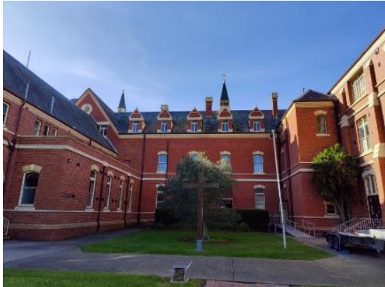
Figure 7: View of the west façade of the original 1893 building. Note that it has been partially concealed by later extensions (indicated in red). Source: Trethowan Architecture, 2023.
