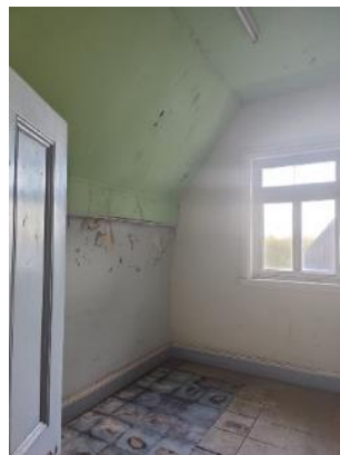
Figure 16: View of one of the dormitory rooms on the second level. Source: Trethowan Architecture, 2023.
