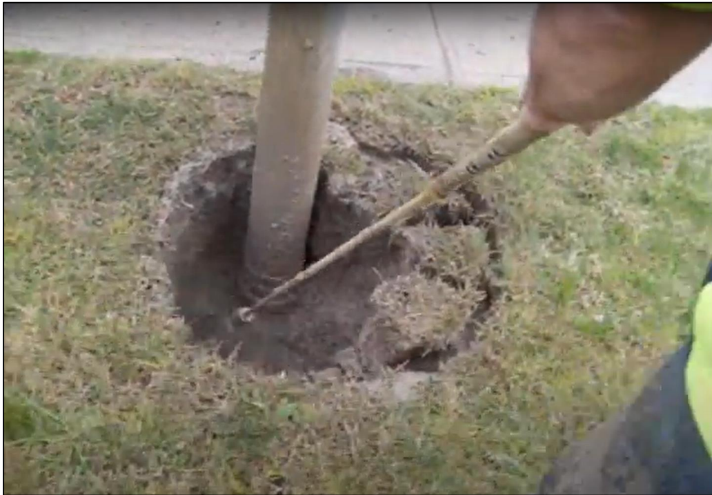
Figure 8. Example of a hole being dug by non-destructive digging methods (NDD). A high-pressure hose is used to liquefy the soil and the soil is then removed by a vacuum. The NDD can be undertaken by one person, which means there is no need for large vehicles to drive over vegetation in the road reserve.
