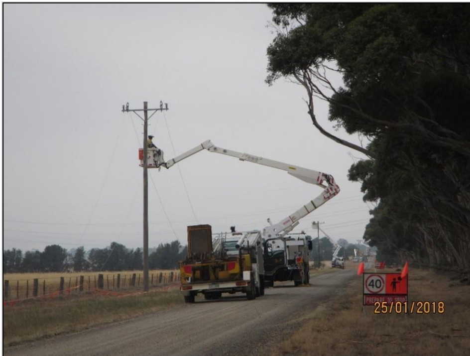
Figure 10. Example of contractors working on a new or replacement pole installation. Note that the truck is still in the road carriageway
