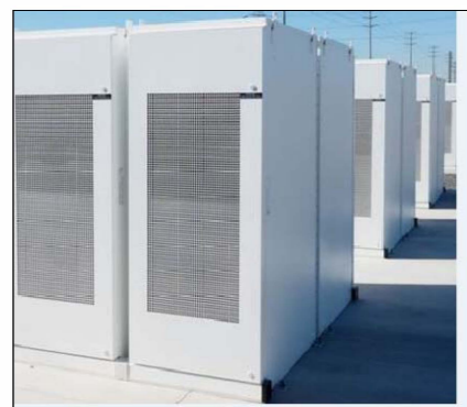
Typical Battery storage unit
