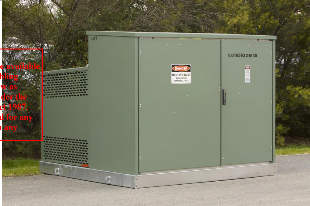
Example of an auxiliary transformer.
