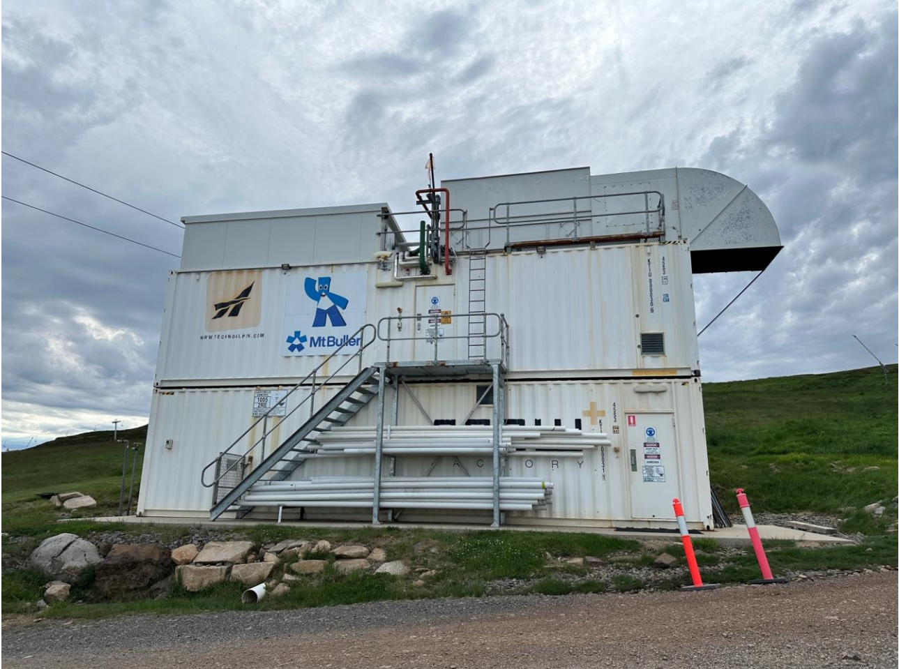
Above: The existing all-weather snowmaking unit installed in 2017 (PA1600151) at the top of the Bourke St ski slope – the proposed unit will be typical of this previous installation
