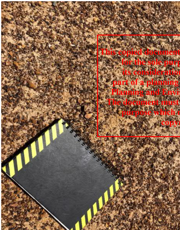
Figure 8: Gravel exposed on farm dam embankment
