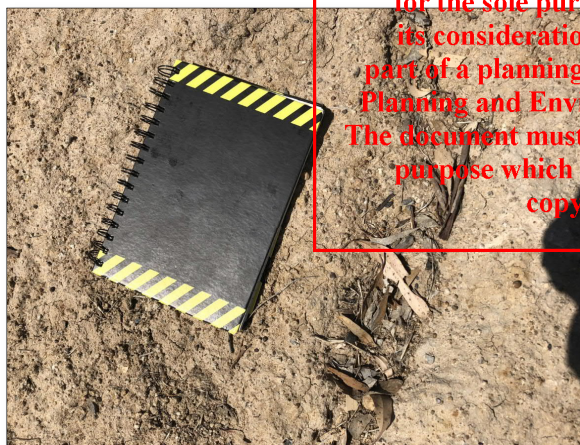
Figure 6: Gravel exposed on farm dam embankment
