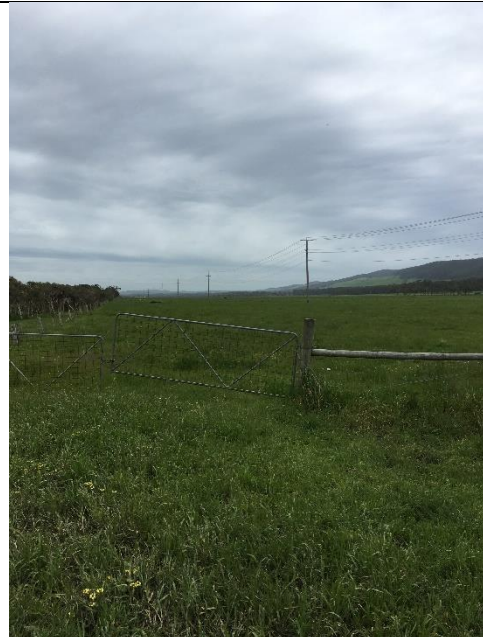
Figure 8 - Existing 66kV power line (right)
