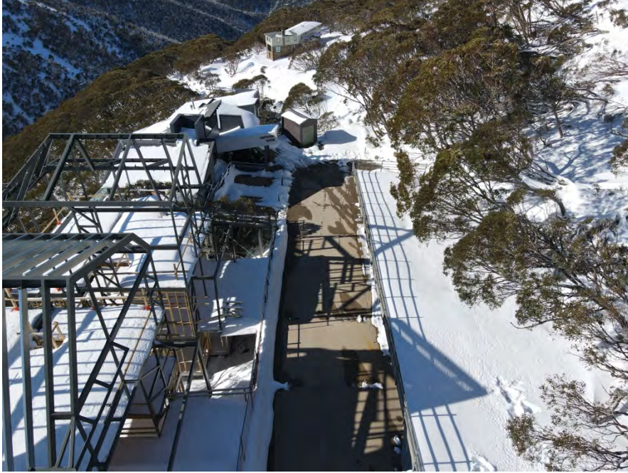
Figure 3.10: Hot Plate Drive looking south east
