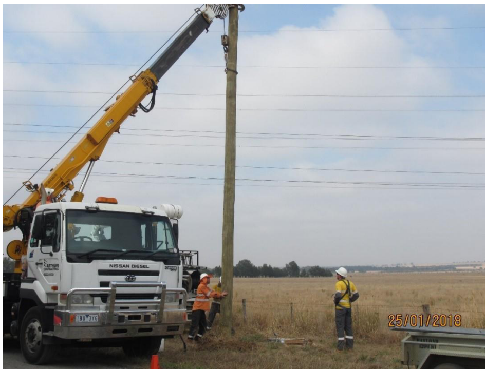
Figure 4: Example of pole being installed via truck crane. Note that the truck can be parked further away if required.
