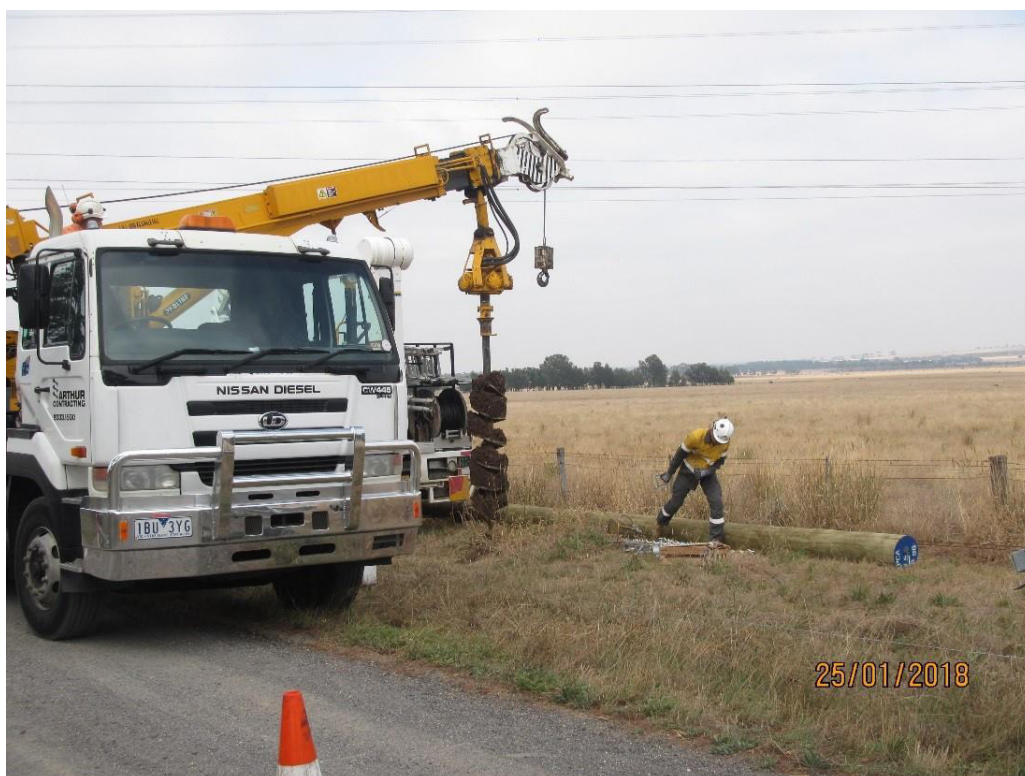
Figure 2: Example of a hole being augured via arm from truck (note in this example the roadside vegetation was deemed to be non-native, hence the truck is parking slightly on the verge and the other truck in the background)
