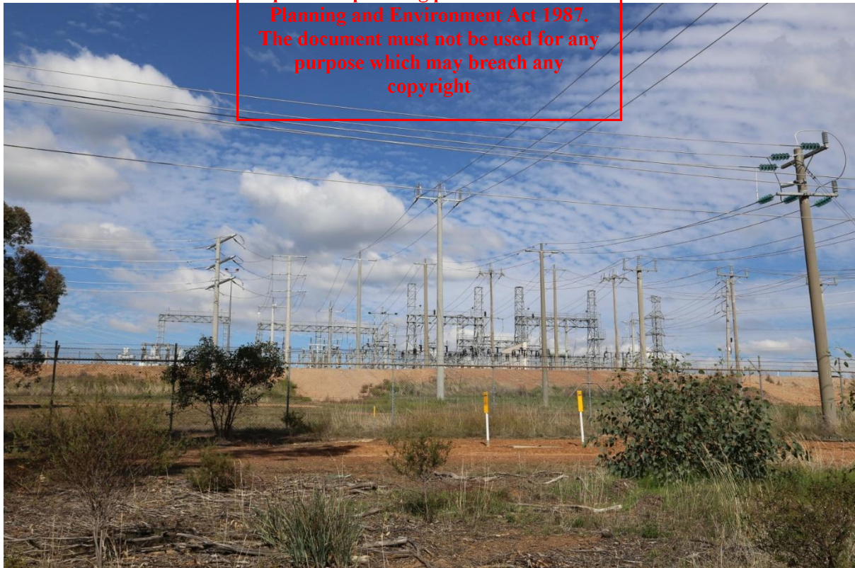
Figure 14 – The Glenrowan Terminal Station, as viewed from Winton-Glenrowan Road.
