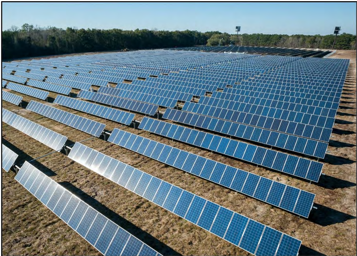
Figure 8. Example of a single axis tracker PV system at 40° angle with reduced inter-row shading.
