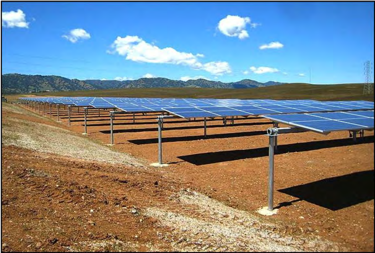
Figure 9. Example of a single axis tracker PV system at 0^\circ with zero inter-row shading.
