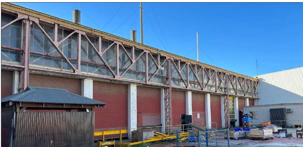
Figure 48 Part the south elevation of the original 1950-52 factory showing the steel truss crane gantry and original roller doors that allowed goods to be taken in and out of the building, and which could also be opened for ventilation in hot weather.
