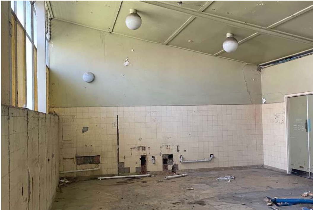
Figure 38 Wash room/toilet inside the amenities block, stripped of most fittings and fixtures.
