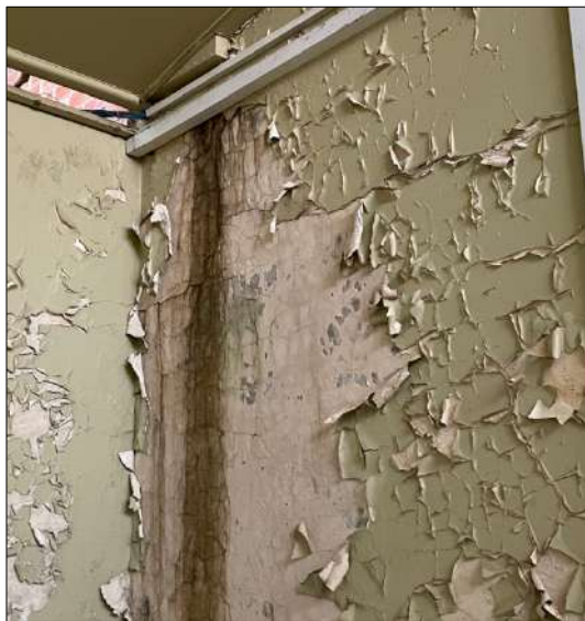
Figure 39 (left) Water damaged walls caused by defective box gutters.
