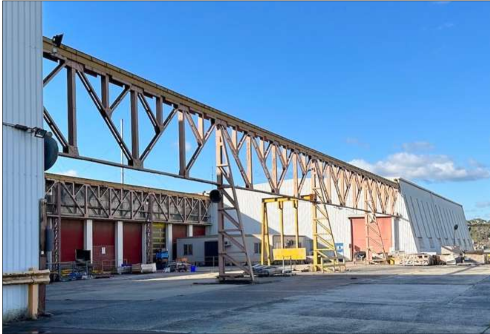
Figure 16 Gantry crane to the south side of the main factory. The structure with the angled wall (to the far right of the image) is a c1984-1990 addition.
